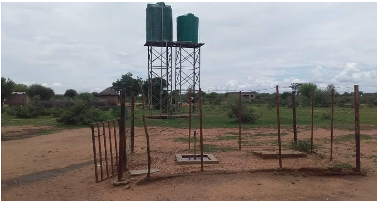
Community-owned water piped tanks in Tshitshi
